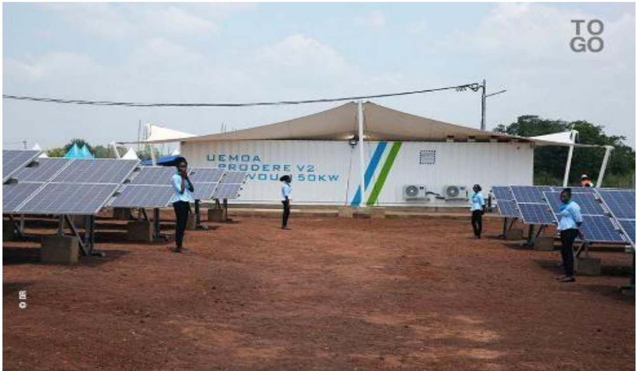
Figure 5: Centrale photovoltaïque de Bavou _Togo
